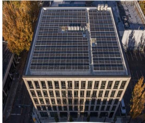
Fig.3.15: The PAE on-site solar array 49
