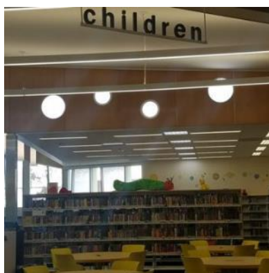
Figure 18 Installation of solar tubes in the ceiling above the bookshelves. This will allow the evenness of natural light throughout the space via the transparent lighting tubes.
