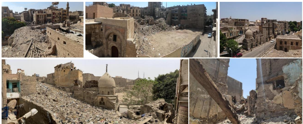
Fig. (6) abandoned and unused buildings, spaces in Darb El-labana area. Source: (Prime Ministry, 2021)
