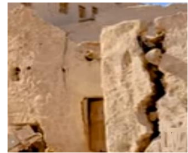
Cracks in Karsheef houses in Shalley, Siwa
