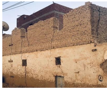
Cracks in mud-brick houses in sharg albalad, Kharga
