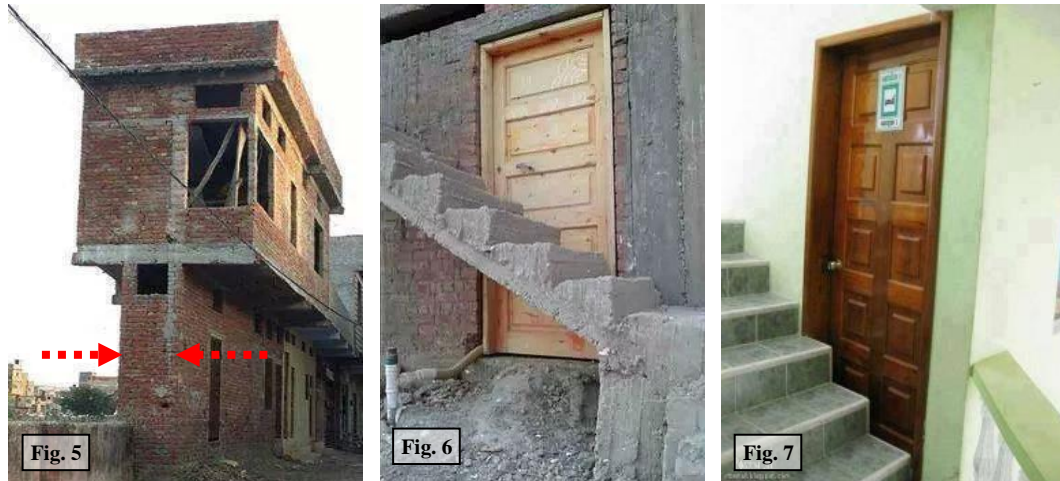
Fig.5→7: Design & Construction mistakes indicating the absence of engineering role, Author.
