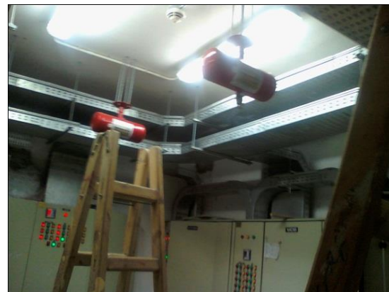
Fig.19: Electrical control panels room in a commercial building, Author.
