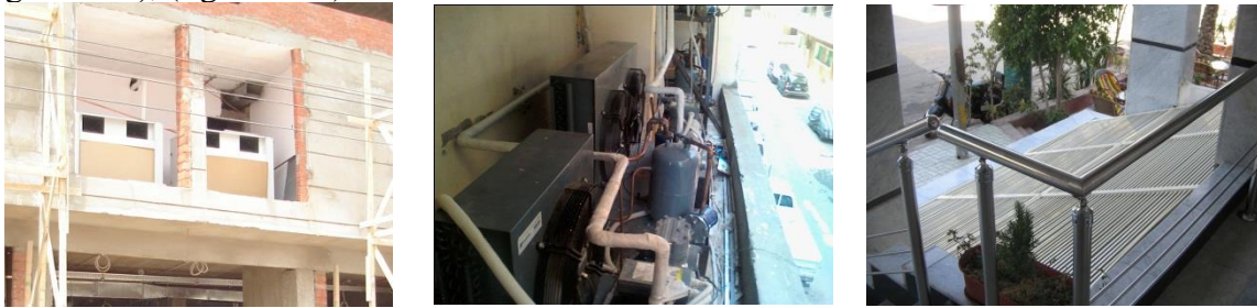
Fig. 15→17: Use recessed open space for external A/C & refrigeration units then hide it with aluminum lovers at elevations of commercial buildings, Author
