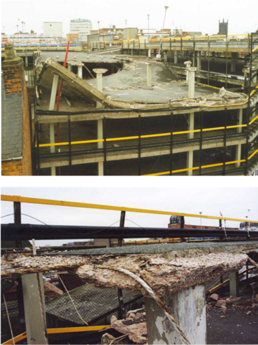
Fig. 2. Punching Shear Failure at Interior Slab-Column Connections - Piper's Row Car Park, Wolverhampton, UK, 1997 (Wood, 2003a, 2003b)
