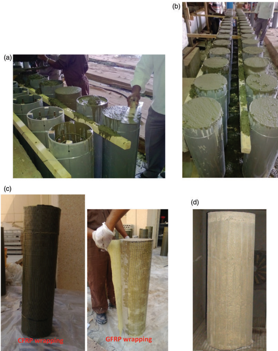
Figure 2. Specimen preparation, strengthening and insulation. (a) Plastic pipe formwork and steel cage during casting; (b) column specimens after concreting and leveling in plastic pipe framework; (c) columns ready for curing after FRP application; and (d) column insulated using Sikacrete-213F.
