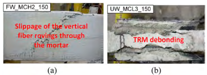
Fig. 28. Failure modes of TRM-strengthened beams tested by Tetta and Bournas [117]: (a) Two layers of fully wrapped jacket at 150 °C; (b) Three layers of U-wrapped jacket at 150 °C.
