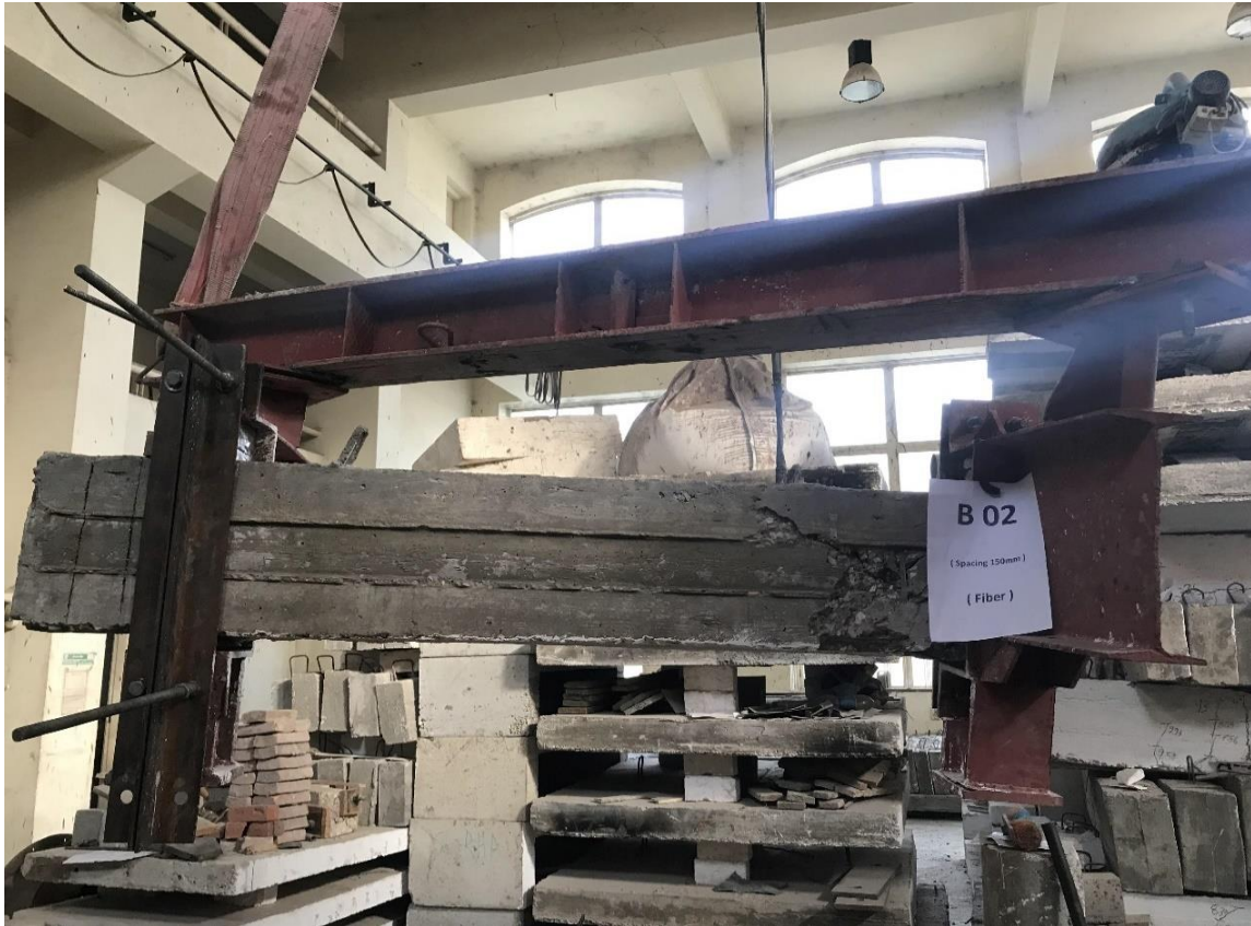
Figure (4-12-b): Cracks Pattern Second Side for Specimen B2.
