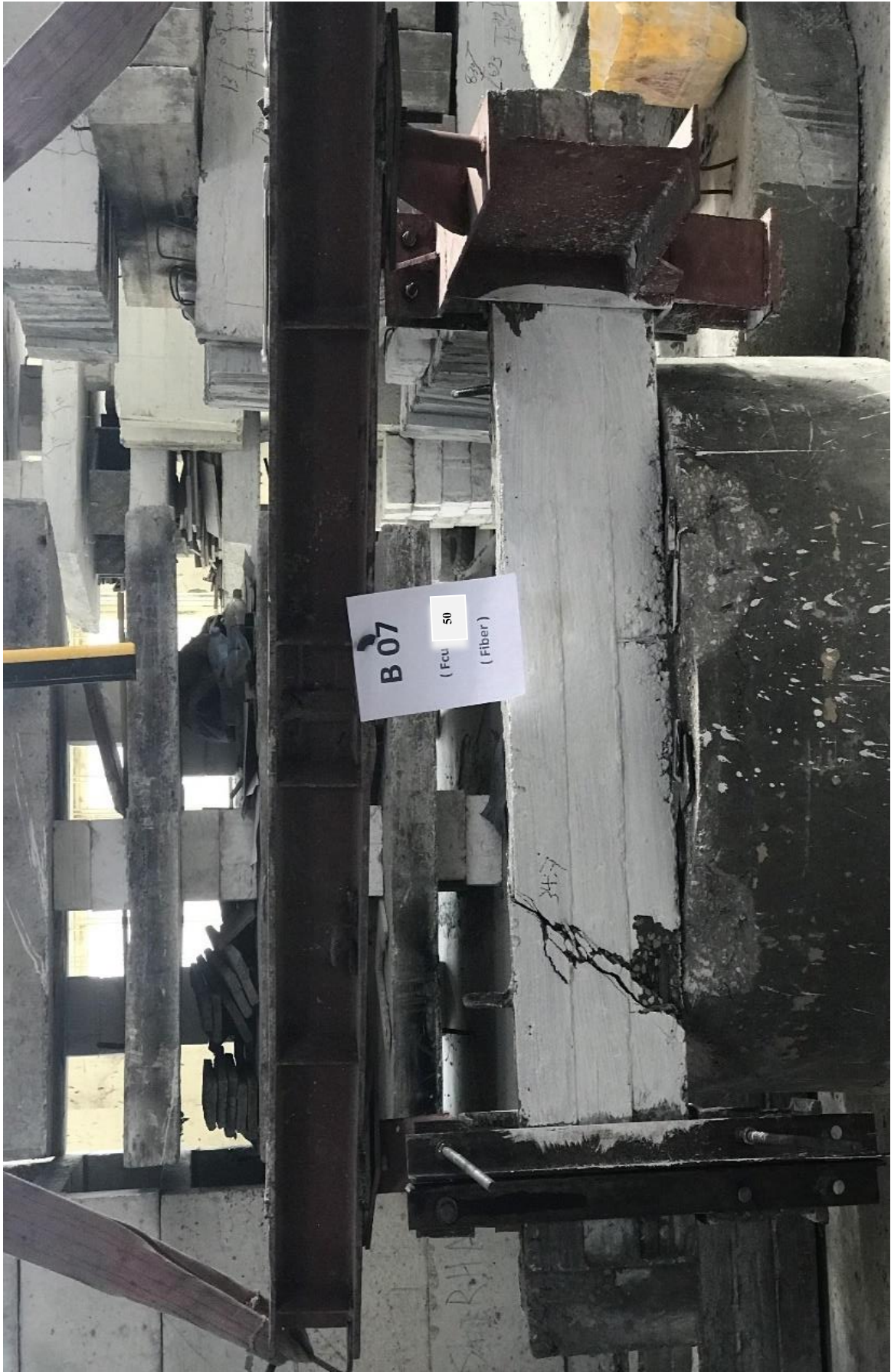
Figure (4-54-b): Cracks Pattern for the Second Side of Specimen B7.
