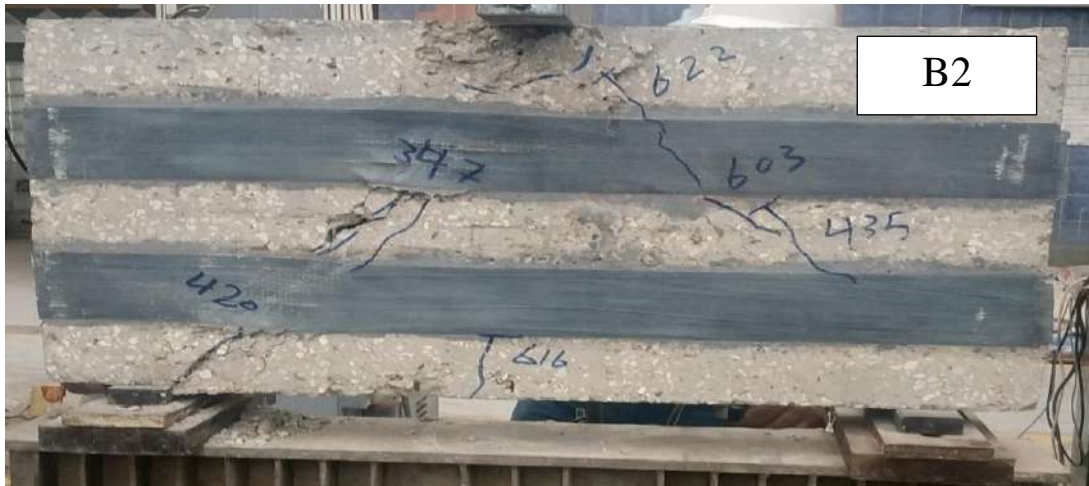
Figure (4-2): Crack pattern at failure (B2)
