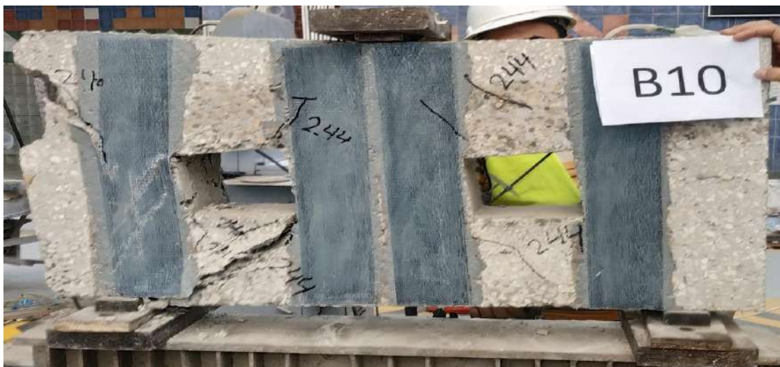
Figure (4-10): Crack pattern of beam B10 at failure
