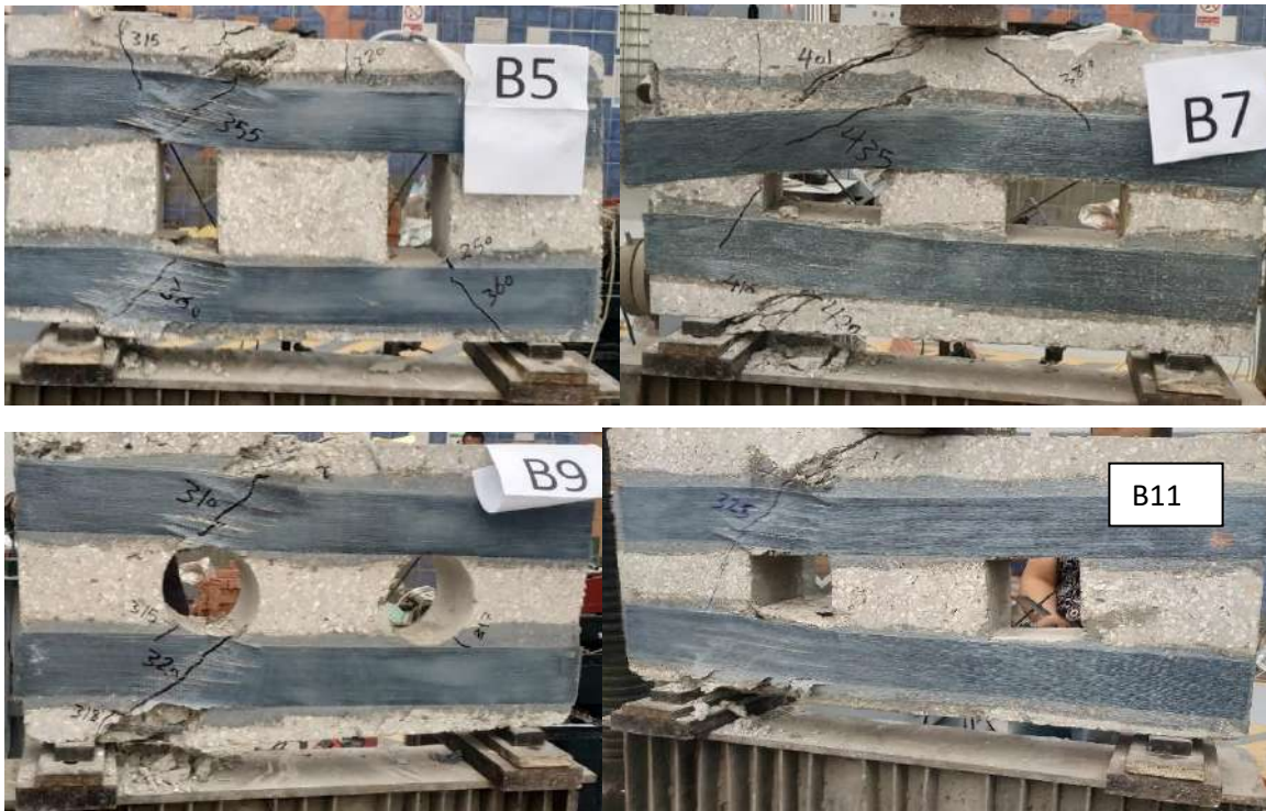
Figure (5-3): Crack patterns for beams strengthened with horizontal BFRP strips.
