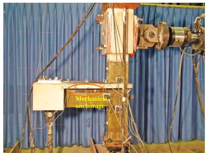
Fig. 8. Photo showing GFRP scheme applied to as-built exterior joint (image by the authors)
