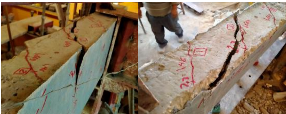
Figure 14 : Cracks Pattern in G2 .
