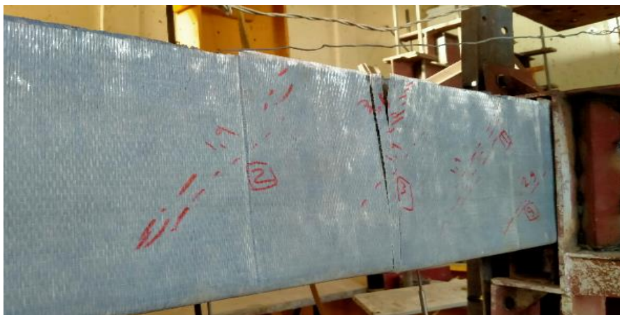
Figure 13 : Beam wrapped around the beam having U-warp for web after cracking (G2).
