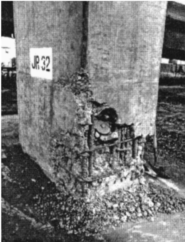
Fig. 2. Brittle bond failure of lap splices at column base, 1989 Loma Prieta earthquake
