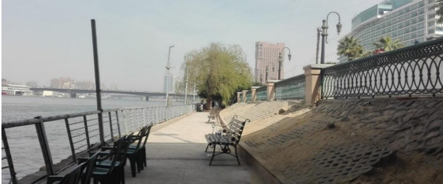
Figure 52: Barren concrete levee extending from the upper promenade to the lower-level with dilapidated structures, broken metal railings, and informal seating areas on the east bank. Source: Author.
