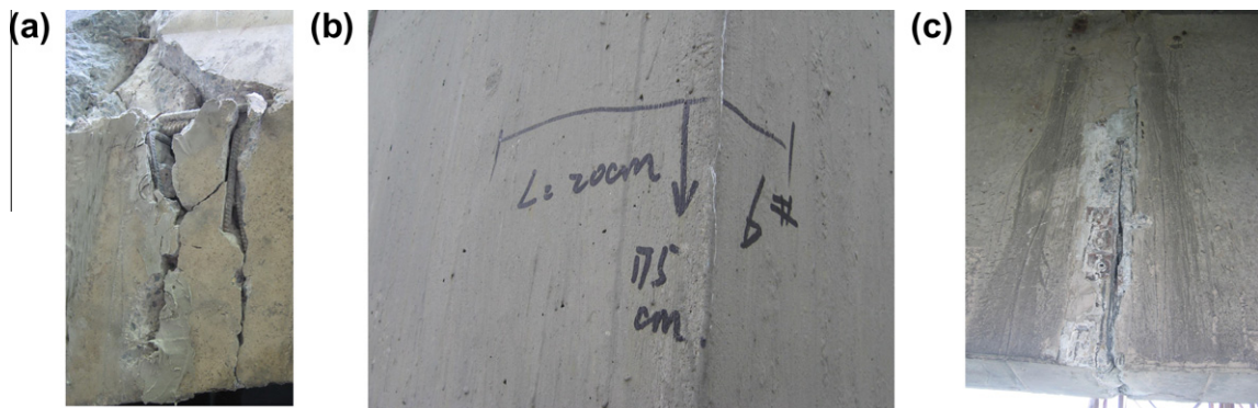
Fig. 9. Cracks shape of (a) Deck near abutment (48.2 m from Tianjin bridge side), (b) Tower, and (c) Deck near mid-span of bridge.
