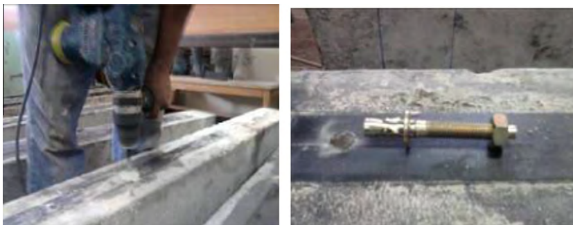
Figure 3 The procedure for fixing and fastening the rivets with CFRP laminate and concrete surface.
