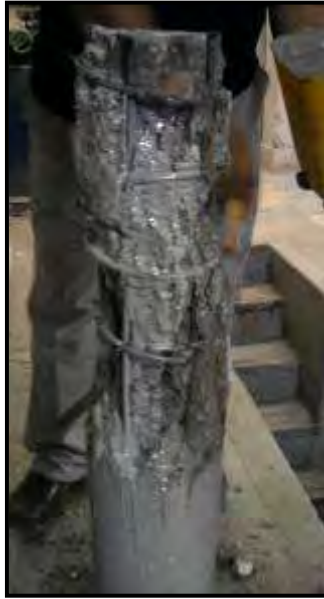
Figure (4) repairing the top part of the loaded column (C3) before strengthening
