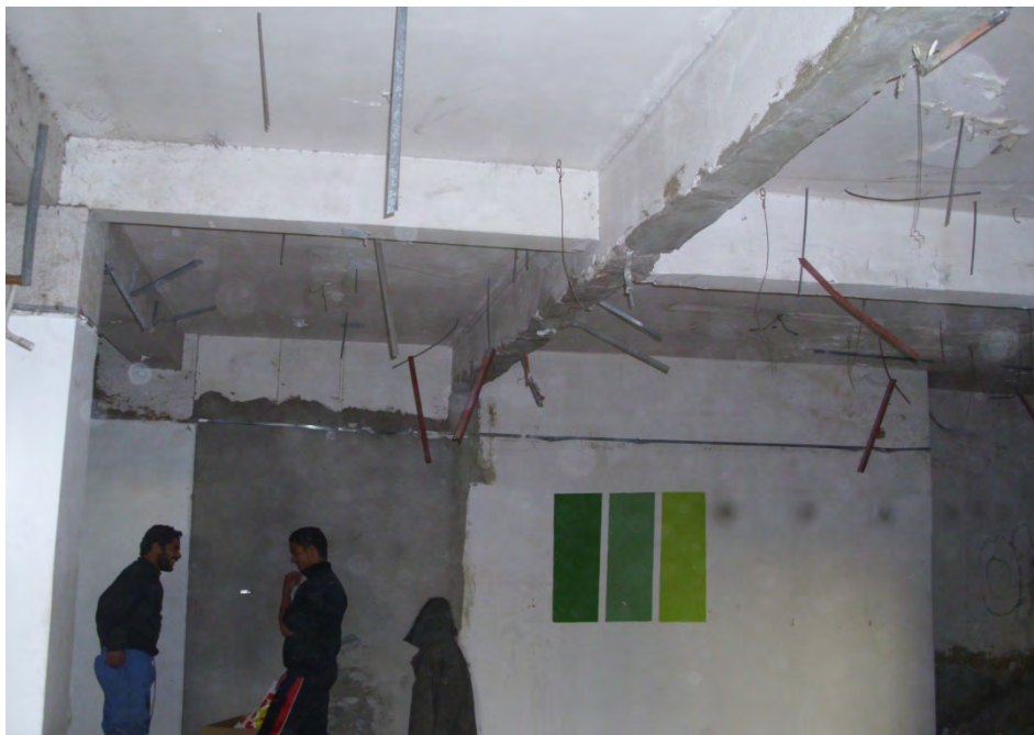
Figure B.4 long span beam with a 55 cm depth only loaded by tow beams.
