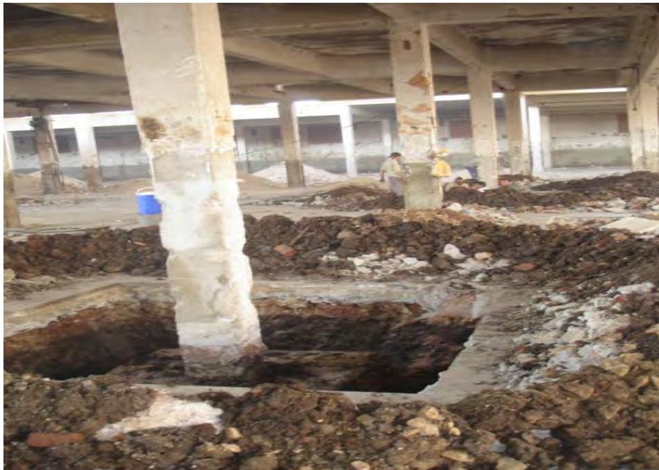
Figure A.7 Excavation around the footing.
