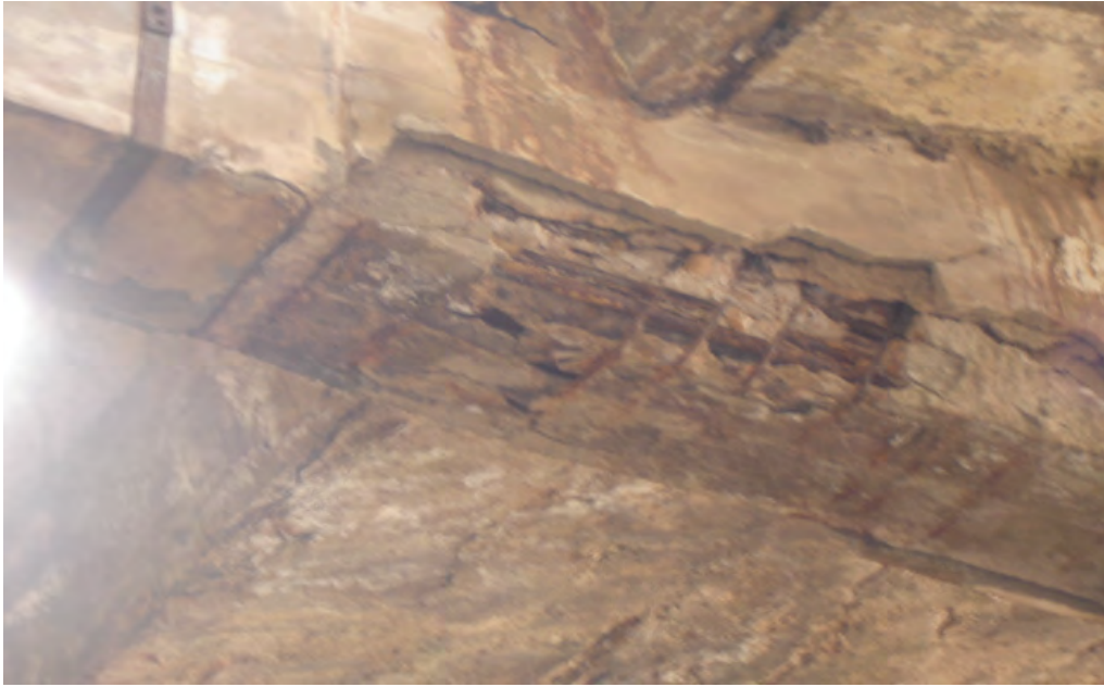
Figure A.19 Damaged girder.
