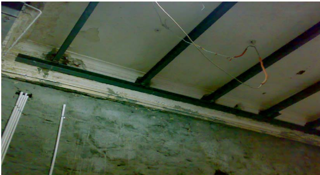
FigureC.9 Damaged slab strengthened by steel beams.
