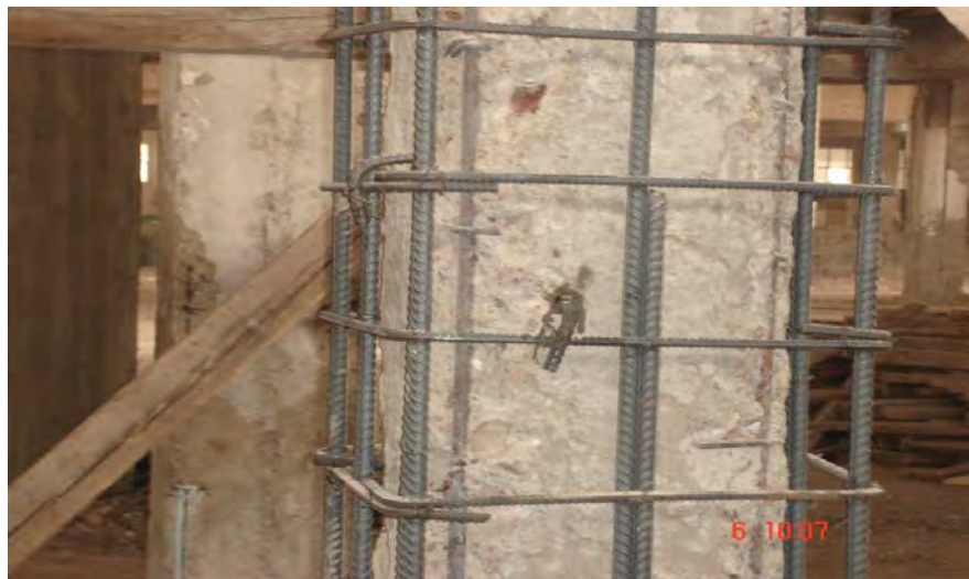
Figure A.13 Rebar's splice between column's jacket main steel and steel dowels planted in the footing jacket.
