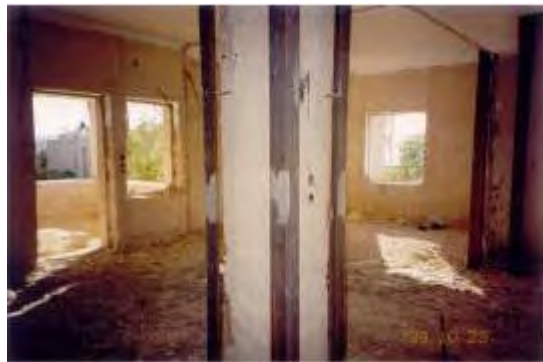
Figure 4.8. shows a column which was strengthened with steel angles
