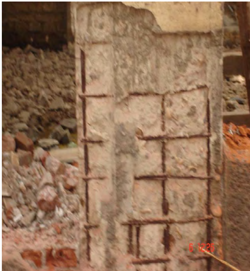
Figure A.33 Damaged column in the first level.
