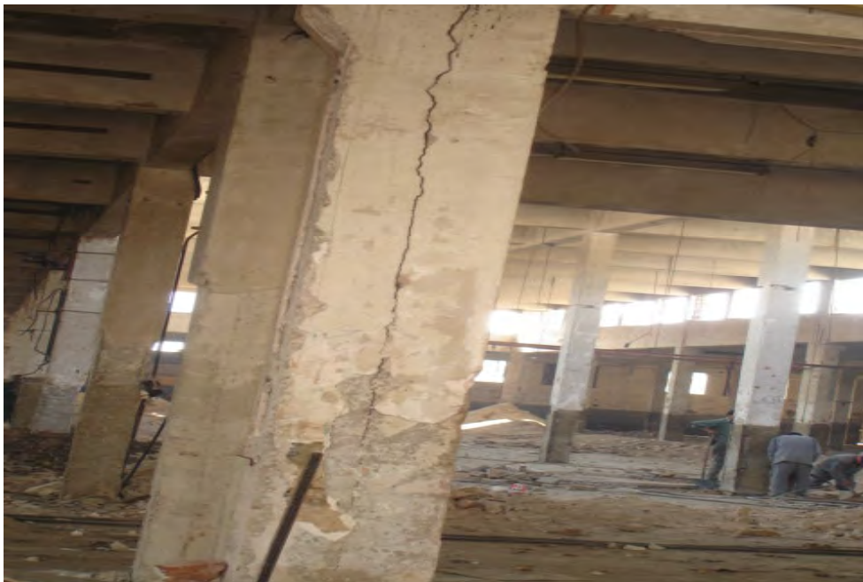
Figure A. 5 Column with longitudinal cracks.
