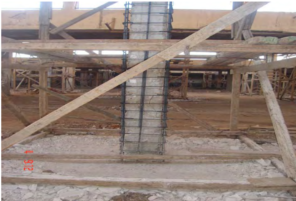
Figure A.11 Completing casting the footing jacket and installing reinforcement steel jacket of the columns.
