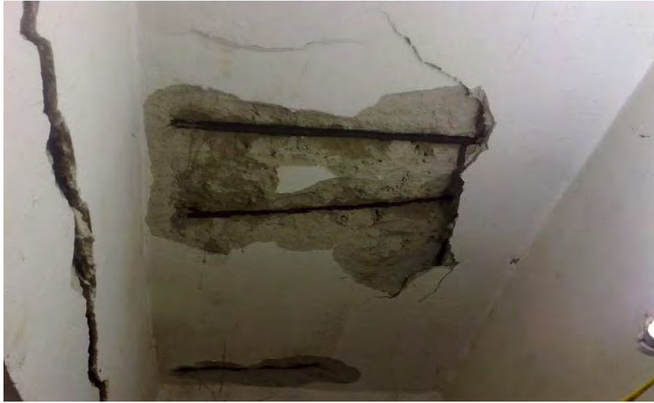
Figure C.5 Damaged beam and slab.
