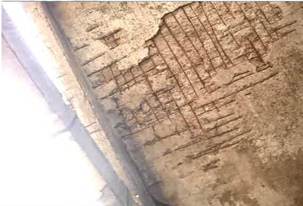
Figure A.20 Damaged slab and girder in workshop (2).
