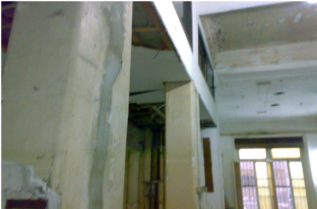
Figure C.6 Two RC columns need strengthening.
