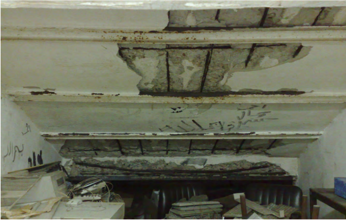
Figure C.3 Damaged stairs slab.
