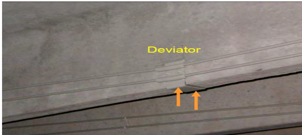
Figure 6.10 Cable deviator added to make a profile similar to the bending moment .
