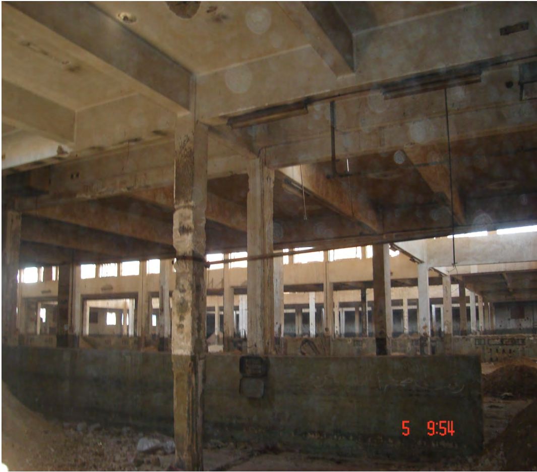
Figure A.6 Columns with clear height of more than 6.3m and a concrete dimensions of 35X35 or less.
