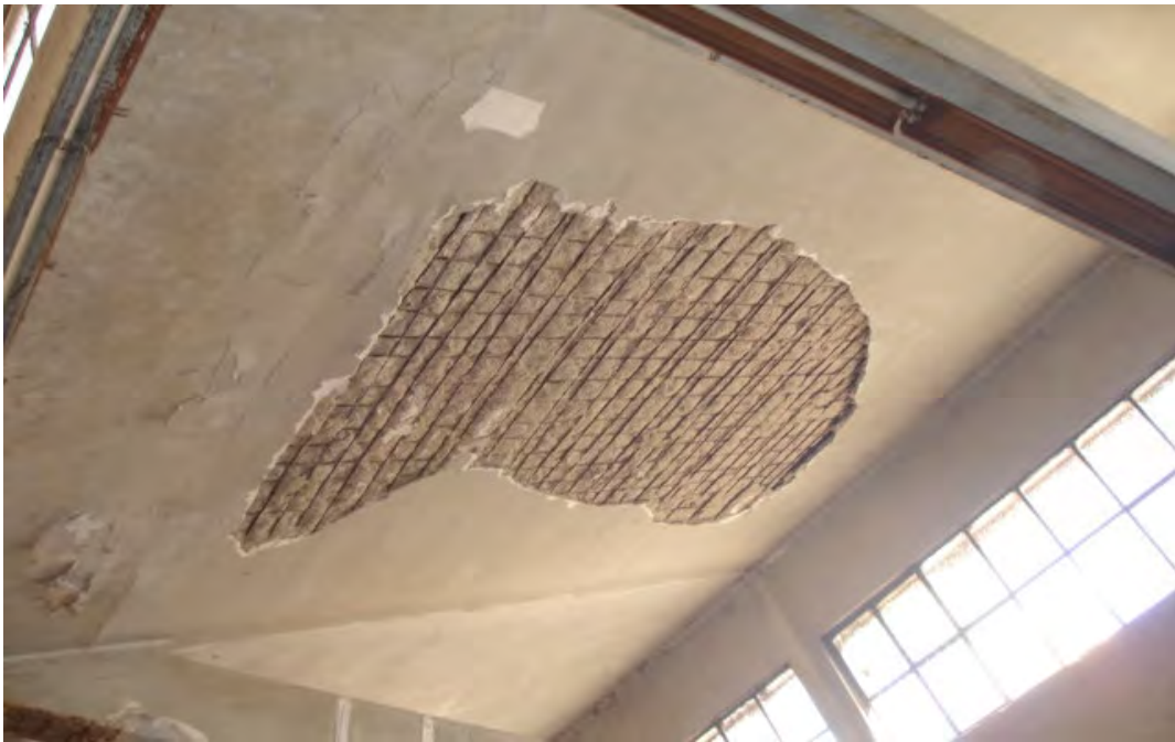
Figure A.18 Damaged slabs in workshop (2).
