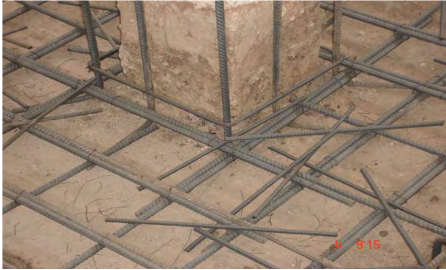
Figure A.10 Interaction between the column jacket steel and the footing jacket steel.
