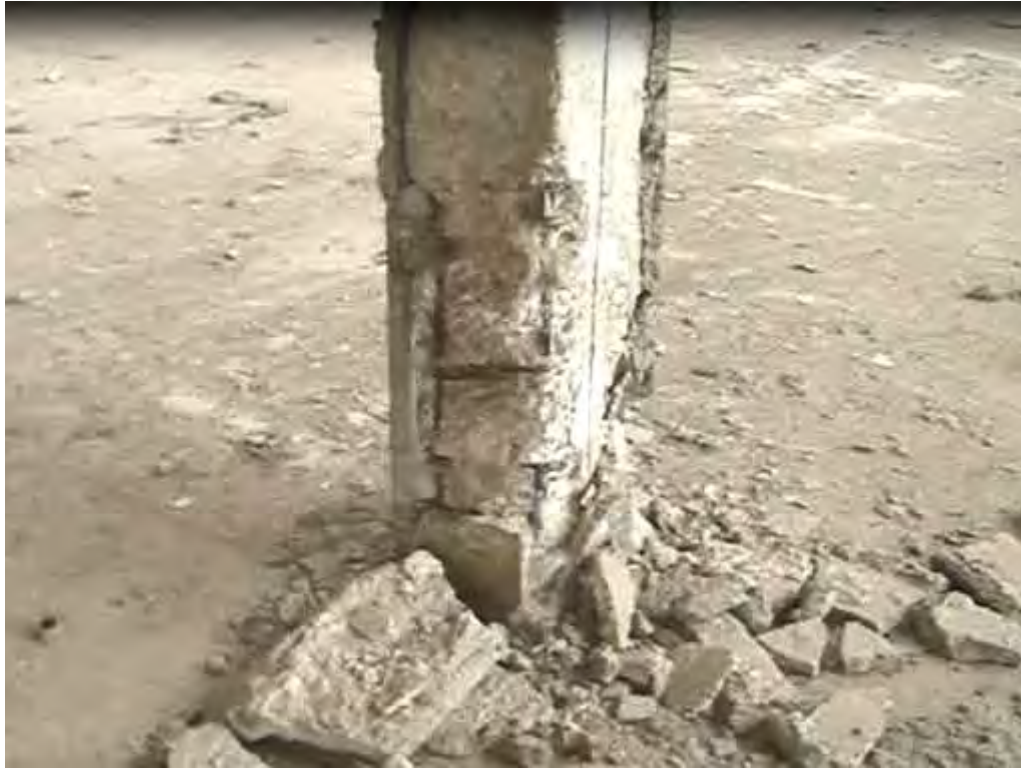
Figure A. 4 Columns concrete damaged.
