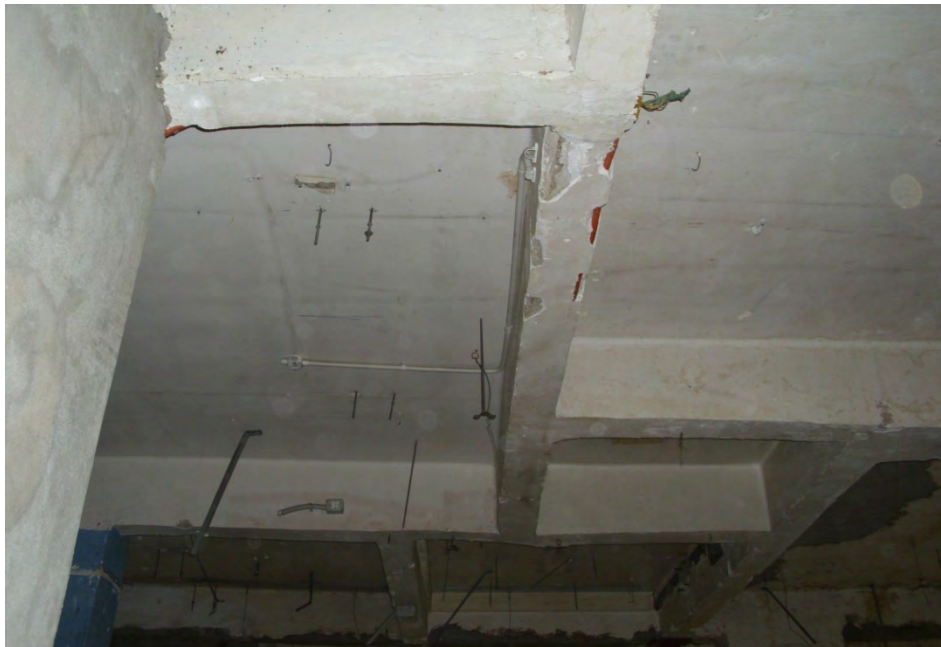
Figure B.3 Very bad beams system.
