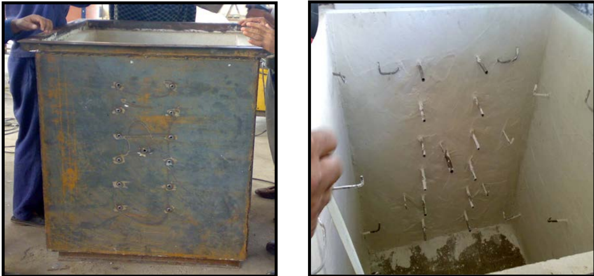
Fig.3.10 Furnace steel skeleton and the stainless steel tubes
