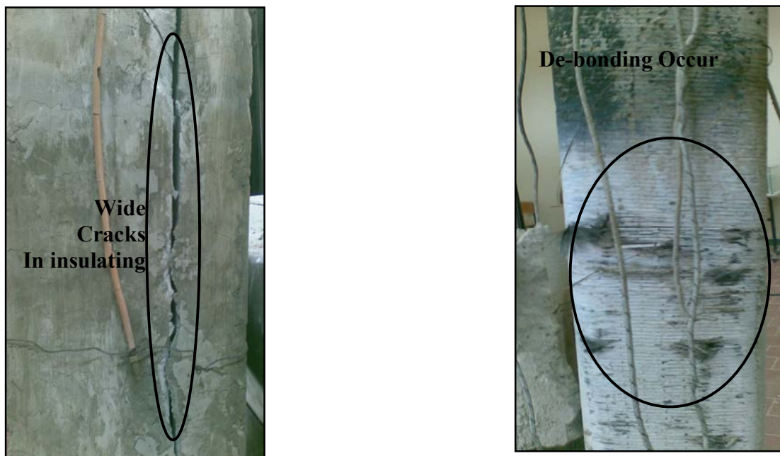
Fig. 4.40 shows the cracks at insulating materials and the bond of CFRP while removing insulation after exposure to 250°C for 24 hours.
