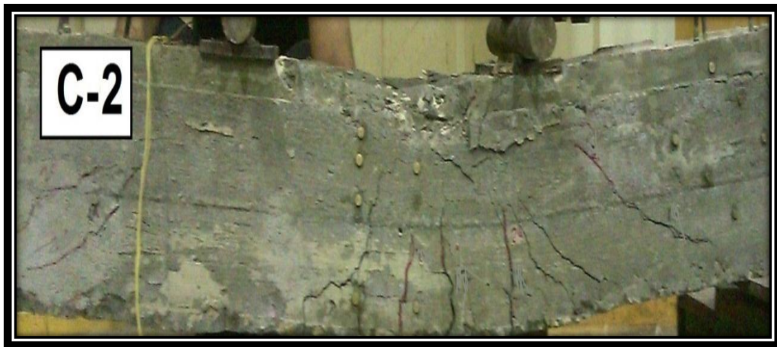
Fig (4.31). Crack Patterns for specimen (C-2).
