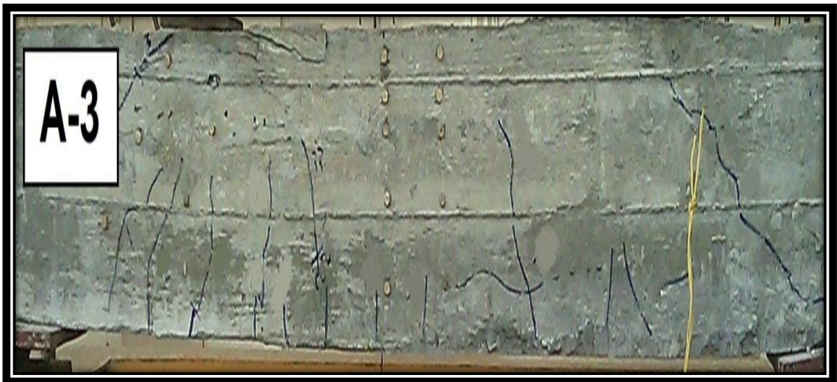
Fig (4.10). Crack Patterns for specimen (A-3).
