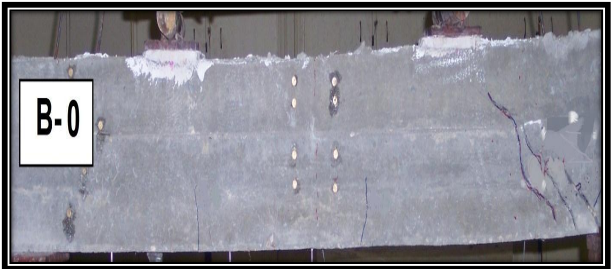
Fig (4.13). Crack Patterns for specimen (B-0).
