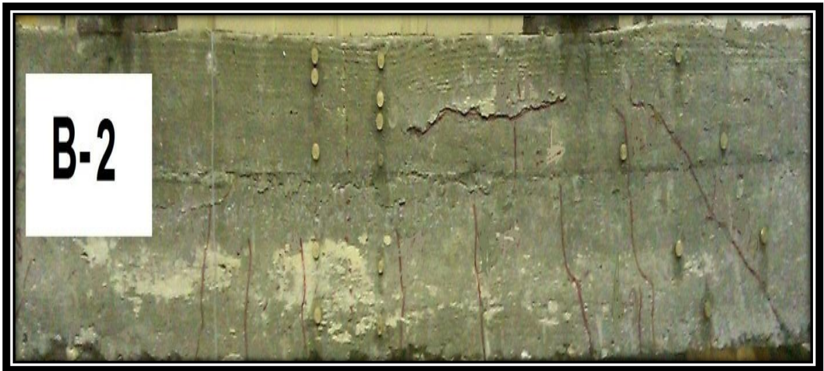
Fig (4.19). Crack patterns for specimen (B-2).
