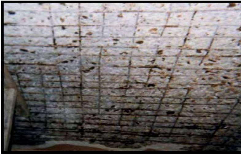
Fig. C-4 Concrete cover is fall from slab.
