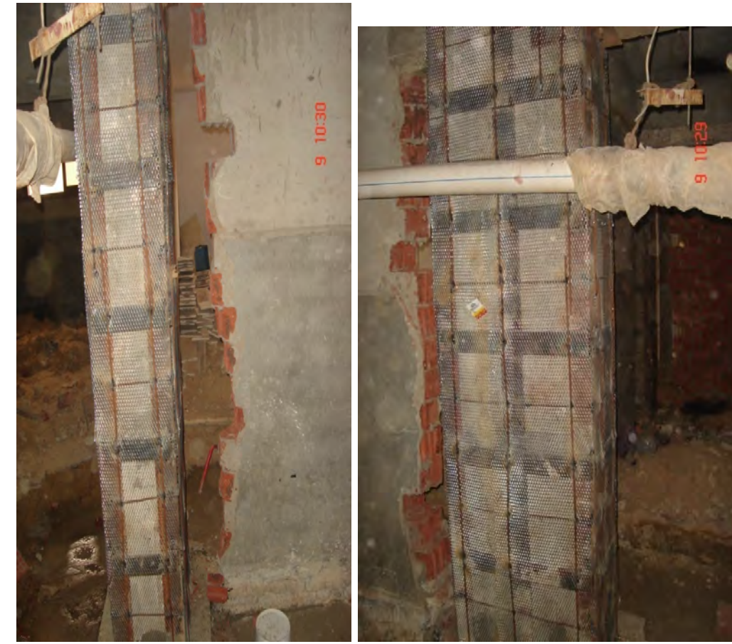
Fig. B-6 column steel jackets
