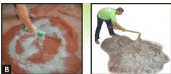
Figure 4. Cement soil mixing according to the Brazilian Standards. Source: ABNT (2012) NBR 10833, NBR 11798 & ABCP (1986).
