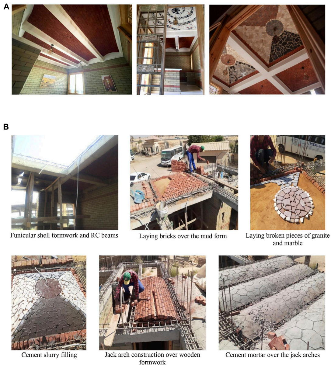
FIGURE 4 EH Alternative roofing: (A) jack arches and ceramic shell in the kitchen and bedrooms (DPLM doors are shown before installing the polycarbonate sheets), and broken marble/granite and brick funicular shells in the LR; (B) parts of the construction of funicular shell and jack arch (Source: authors).
