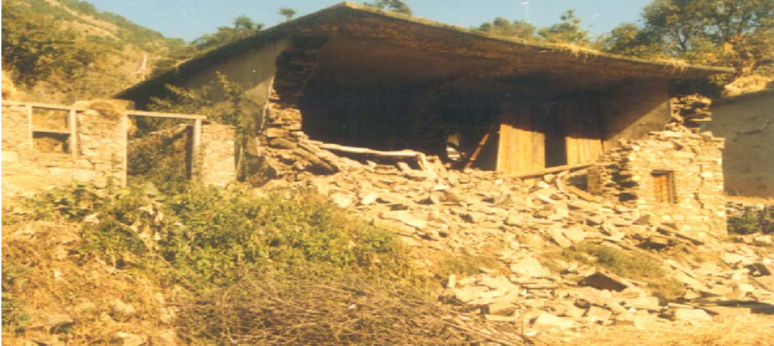
Figure 1.13-Partial collapse of stone masonry walls during 1991 Uttarkashi (India) earthquake.
