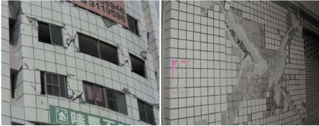
Figure 1.25- Typical shear failure, Chi-Chi Earthquake in Taiwan
