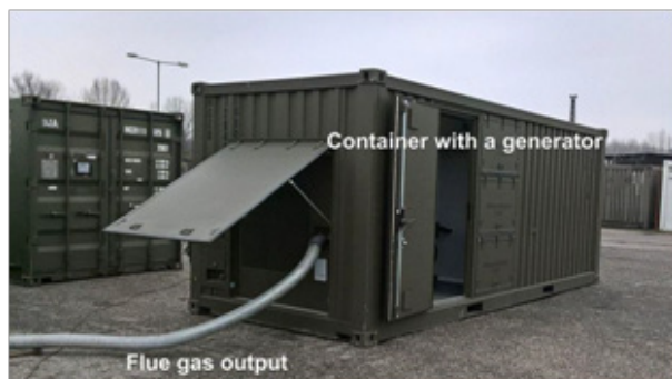
Fig. (3a): Electricity generator inside a safe container in military base camp
