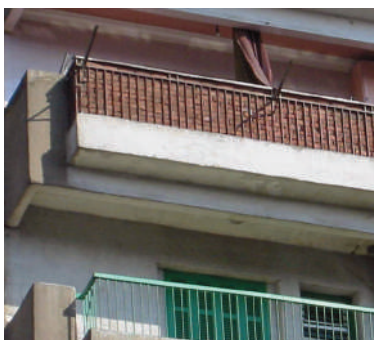
Fig.32. Modifications of the railing. The railing is closed with a cloth or with bricks to preserve privacy while sitting in the balcony. Above, apartment in 15th May City ( www.e-dar.com ); below, apartment in Imbaba (the author).
