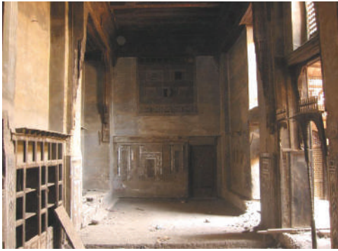
Fig.51. Second floor's qa'a overlooked by the upper qa'a 's mashrabiyya , Bayt Shabshiri (Islamic Art Network)
