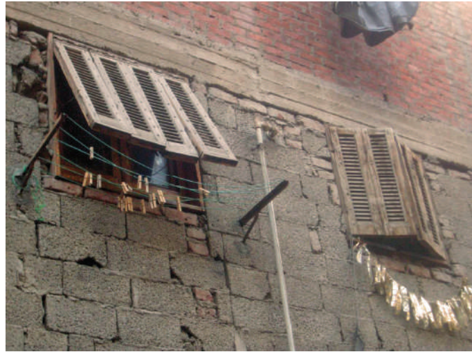
Fig.38. Changing the opening direction of the sheesh from sideward to upward to preserve privacy while hanging the washing. Note that the other sheesh (without washing lines) has not been changed. (The author)
