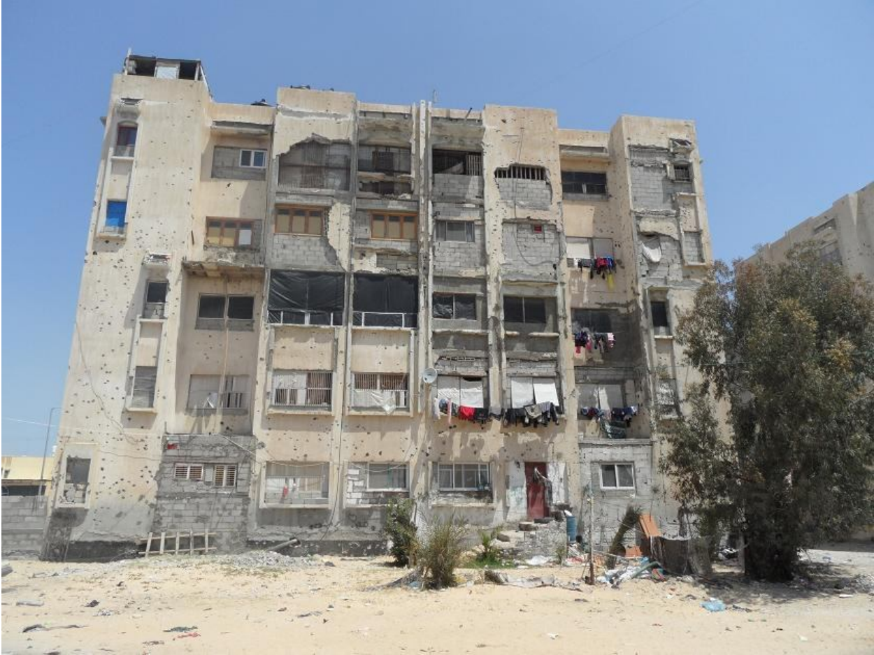
Figure 3.2: A partially damaged housing project with multi story buildings.
