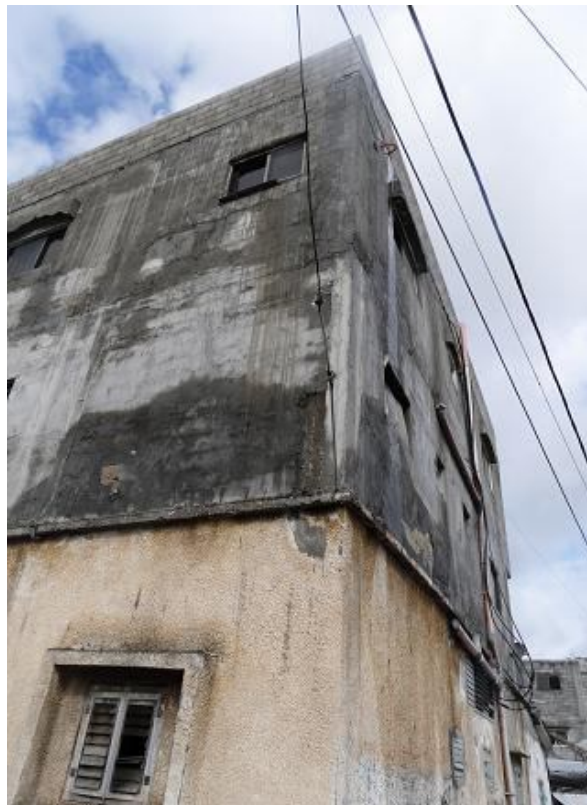
Figure 3.3: A typical self-built house in the Gaza Strip where form is dictated by needs of occupants.
