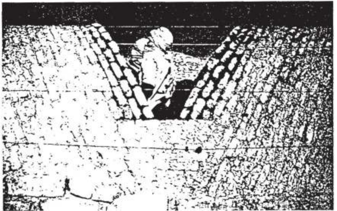
Double-ended vaults being built in Niger. Horizontal courses fill in the tight gaps between two approaching vaults. The masons work with guiding horizontal strings to ensure good vault alignment.
