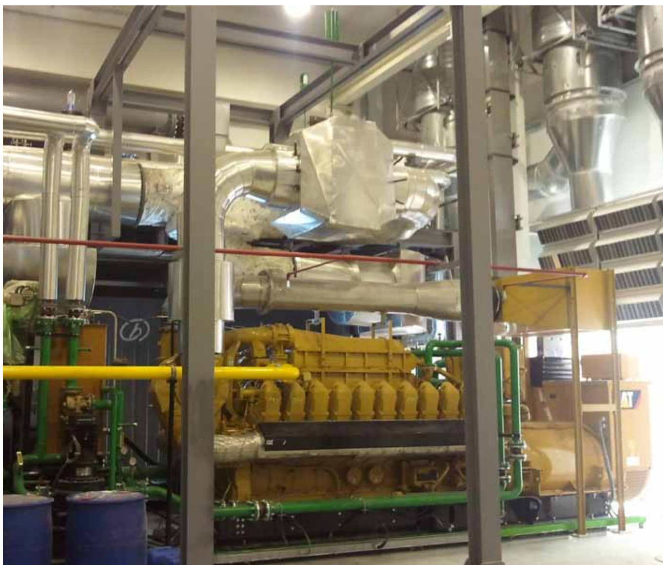
4 MW Tri-generation system, Enfidha-Hammamet Airport, Tunisia. Investment of 5 Million EUR, including a 20% grant from the Energy Transition Fund
