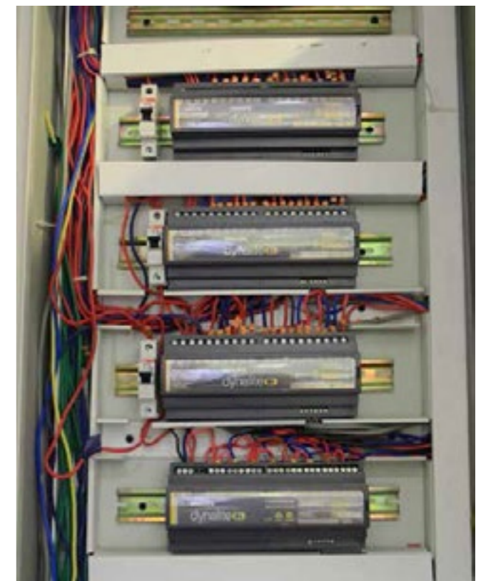
Complex lighting management system at Philips headquarters in Cairo
