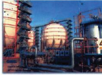
Tanks of Liquid petroleum gaz. (Spherical tanks)
