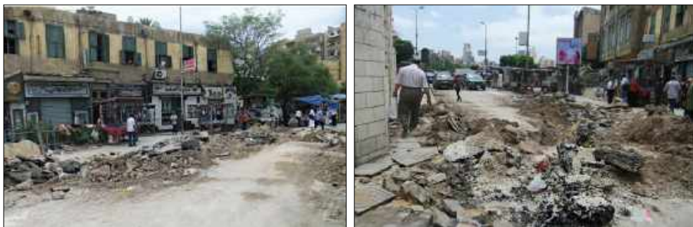
Fig (90): Excavation works for sewage pipeline installation in streets of Alexandria, June 2013
