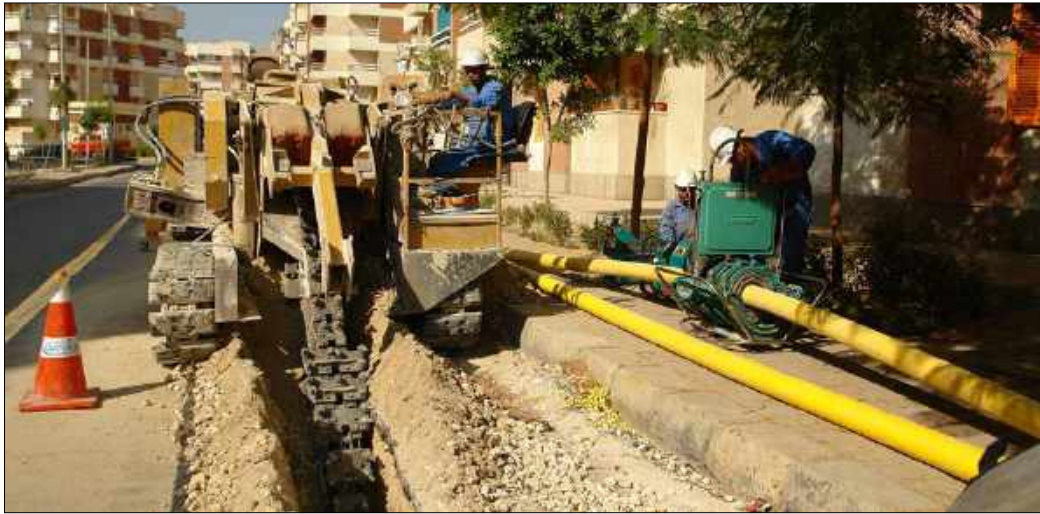
Fig (139): Installing NG lines under the street even with sidewalks available, October city, August 2012
