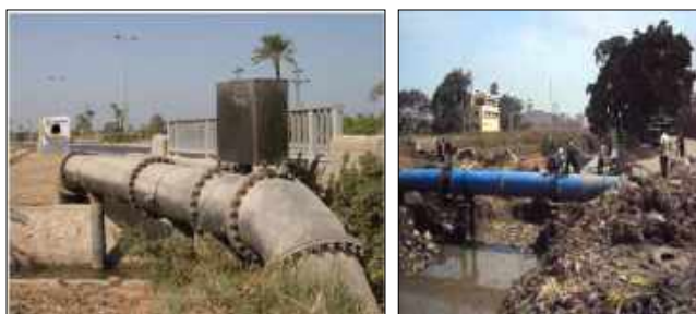
Fig(88): Pipes passing over waterways and leaking occasionally In Kafr Hakim, Geiza.
