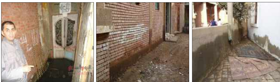
Fig(59): (left) Sewage flooding in rural houses in Al-Tall village, Giza- (Middle & Right) High groundwater table affecting the structure of houses in Al-Khadra village, Menoufia.
