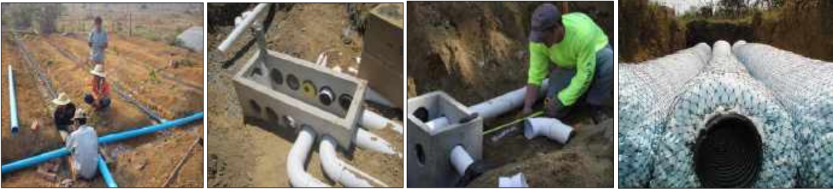
Fig(178): (a) Installing leach field system (b&c) Distribution box installation (d) Polystyrene gravel-free leaching system
