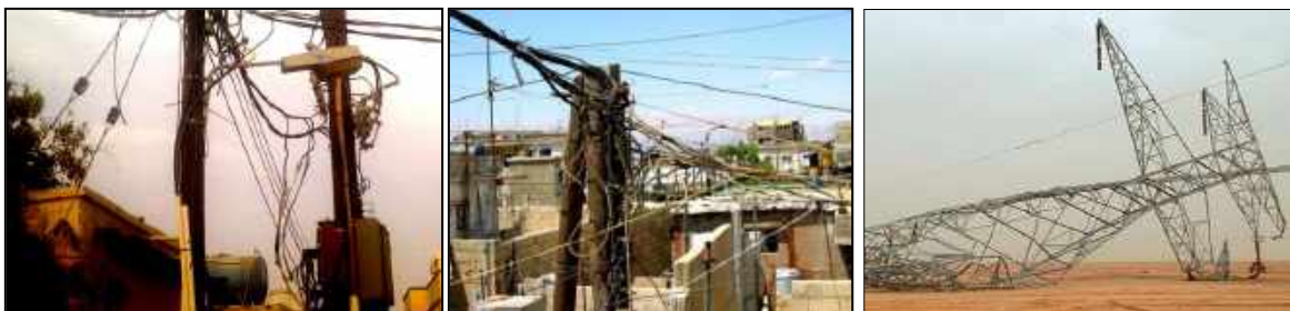
Fig(99) : (a&b) Deteriorated conductors and un-insulated cables in residential districts in Kerdasa and Bahtem (c) Electrical Tower falling by storm in Alwadi-Algedid governorate, March.2014
