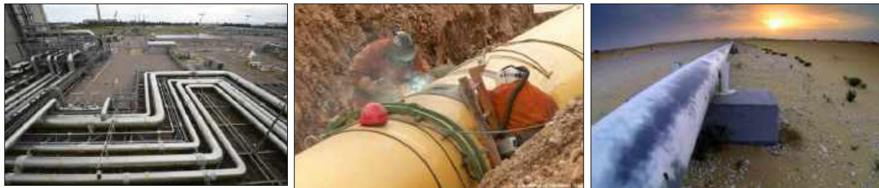
Fig (137): Installing main pipelines for NG above & under ground level in Egypt
