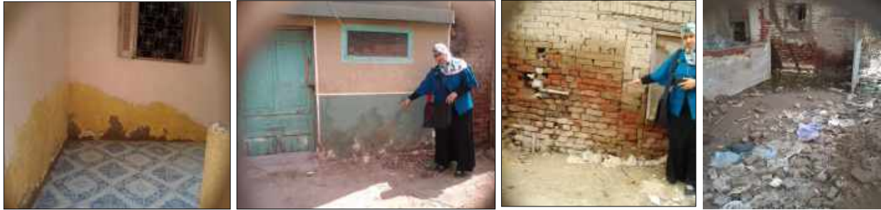
Fig(249): The researcher pointing at wall dampness in Beltag's houses
