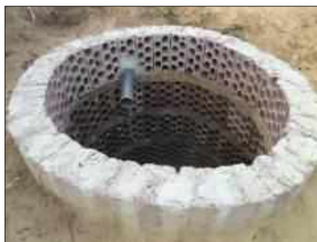
Fig(328): Leaching system built in site with local materials- cavity will be filled with gravel and clean aggregates Source: Ref. No.11
