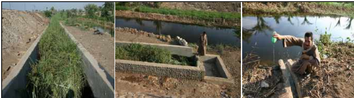
Fig(194): 500 meter of constructed wetland system applied for wastewater treatment, BeniSuief, Egypt
