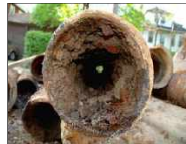
Fig (47): Water pipes clogged by sediments.
