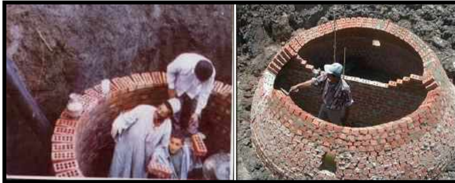
Fig (206): Building Anaerobic Digester chamber in rural Egypt for both blackwater and animal waste treatment
