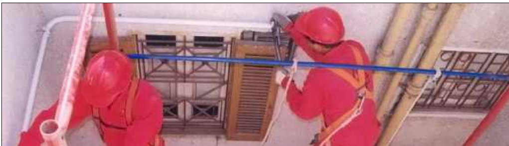
Fig (131): Installing natural gas pipes require good construction status in served buildings
