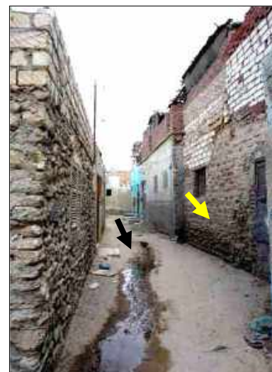
Fig(271): Wall dampness and sewage overflow in Trench-serviced areas in Natroun city
