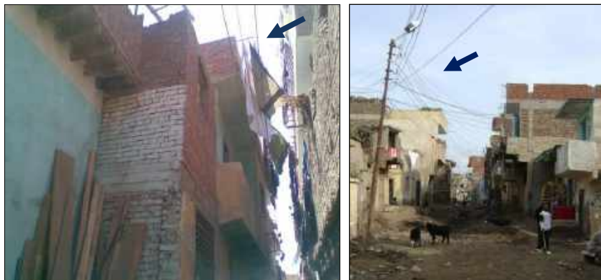
Fig(250): Electric cables so close to buildings in Beltag (left) and entangled electrical cables in Beltag (right)
