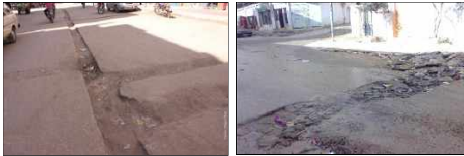
Fig(140): Damaged streets due to delay of restoration after N.G. network installation in Qena (right) and Sheikh Zayed (left). (1)&(2)
