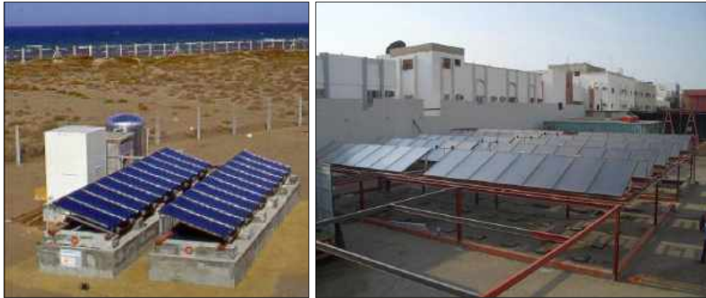
Fig(156): Solar desalination systems applied in Mascat, Oman (left) and Jeddah, Saudi Arabia (right) http://www.solarthermalworld.org/sites/gstec/files/MAGE_WaMa_Intersolar_2010.pdf (left) http://www.dwc-
