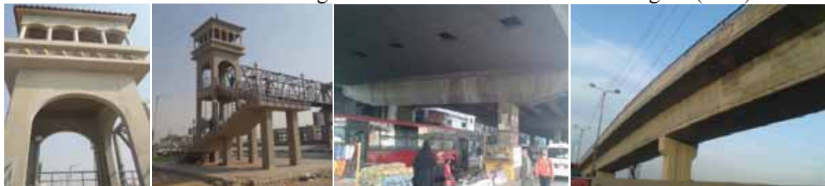
Good concrete quality at pedestrian bridge - Cairo Alex road Bad concrete quality - 6 th of October bridge Bad concrete quality - new constructed bridge - Dumitta
