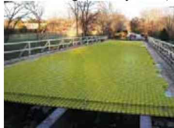
Fiberglass-polymer composites form the core of a renovated bridge deck in Springfield, USA 4
