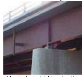
Deck drain hidden by the wing-wall does not have to match the girder color
