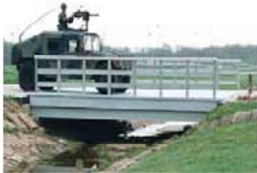
Vehicular bridge at Fort Leonard Wood, Missouri built in 1998 with a maximum load capacity of 12.5 tons.
