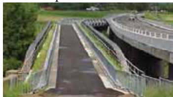
In this adaptive re-use of an old bridge, the wrought iron lattice truss bridge was duplicated and incorporated into an adjacent cycle way
