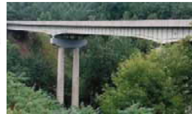
This good example of a hunched girder makes structure looks slender Baltimore
