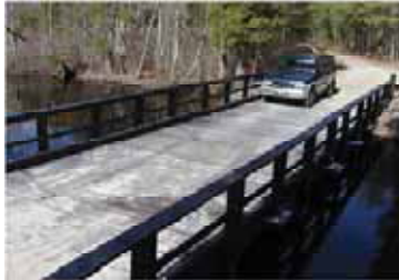
Vehicular bridge in Wharton State Forest, New Jersey built in 2002 with an I-beam substructure and a maximum load capacity of 36 tons.
