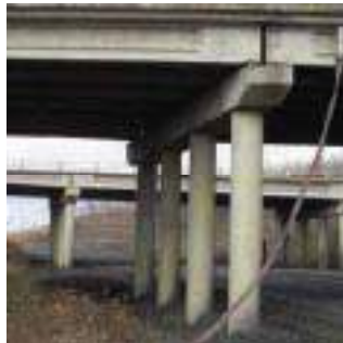
A better attempt needs to be made to conceal the deck to grade drain
