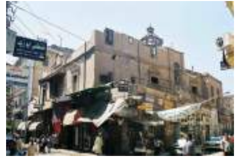
Fig (4-51) The heritage building of cinema Riex is in partially damaged condition Source: (Researcher)
