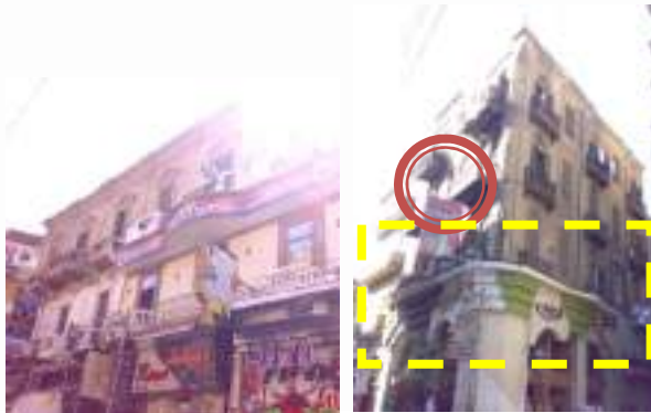
Fig (4-109), fig (4-110) some inappropriate modifications and signs on the facades of the heritage buildings Source: (Researcher)
