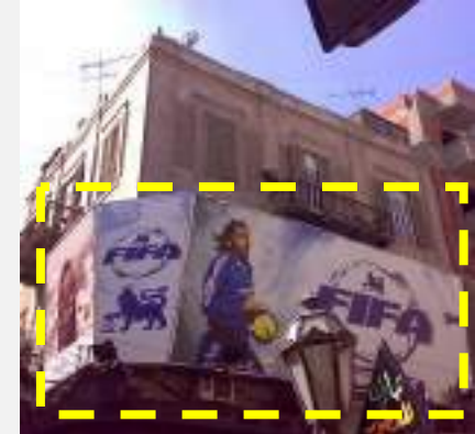
Fig (4-112) The Inappropriate shop's signs, which hides the architecture details of the heritage façade of the building. Source: Foda& Abo-lila(2010)
