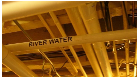
Fig (4-10). River water tubes of the Mansion
