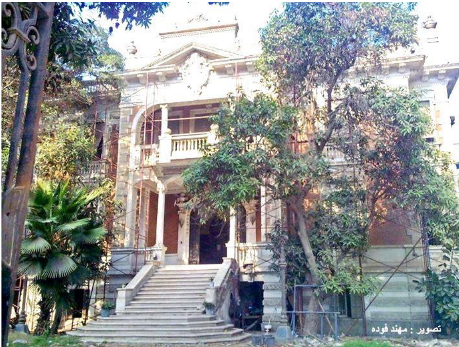
Fig (6-21). The main facade of El-Shenawy palace after installing Metal scaffolding in January 2013.
