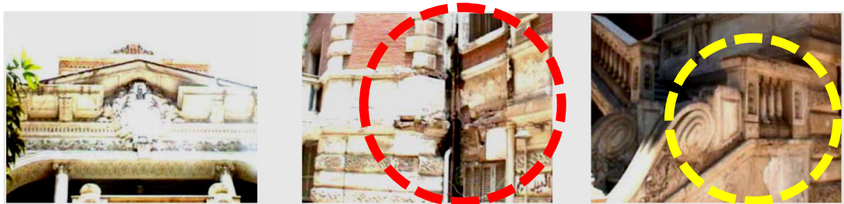
Fig (6-26). The deteriorated parts on the facades of El-Shenawy palace
