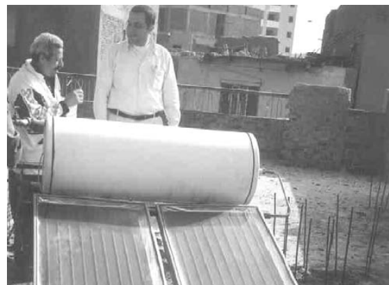
Fig. 2-99 Solar Heating System on Houses Roof, One of the Successful Solar Thermal Systems Installed In Upper Egypt
