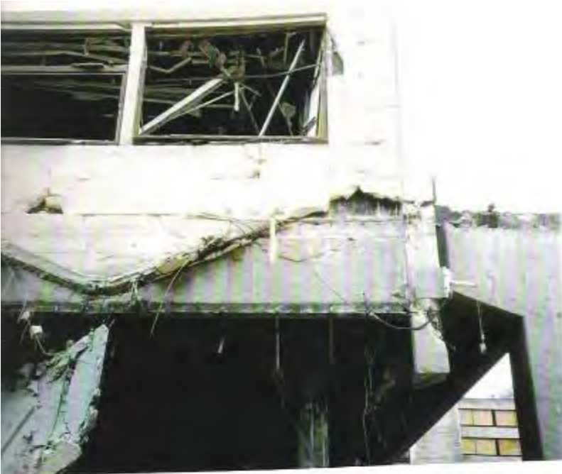
Figure 2.14 Precast concrete panels damaged, Marks and Spencers, Manchester, UK.
