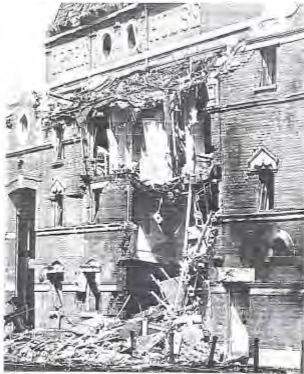
Figure 5.34 Grand Opera House, Belfast: some load-bearing masonry walls are unstable, while others remain relatively intact, an example for masonry wall structure failure, ( Mays and Smith, 1995 ).
