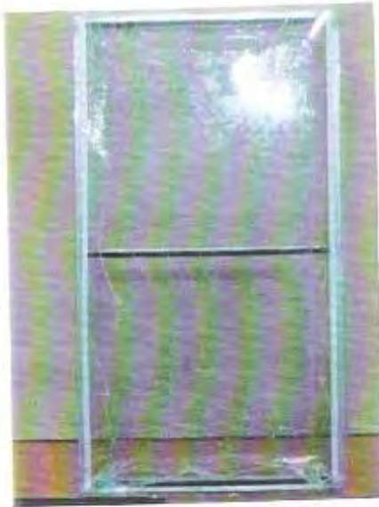
Figure 8.11 One single pane of glass rested on aluminium frame, thin sheet element of aluminium used to support the glass in the middle of the pane.
