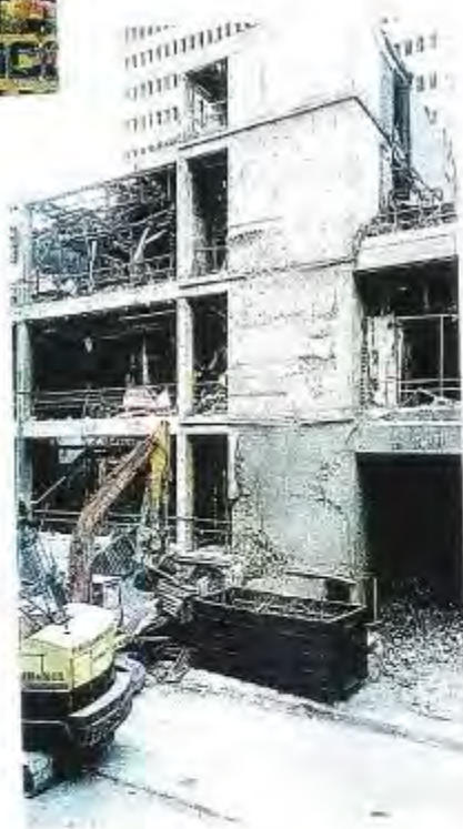
Figure 2.13 The multi storey garage cladding was severely damaged.
