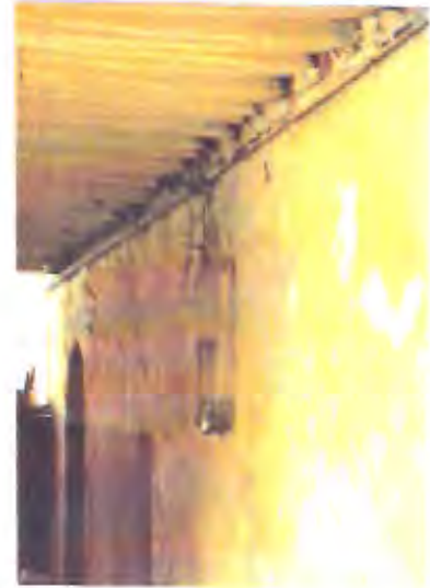
Fig.8-14, Right, inadequate installation for water supply and drainage leading to damp stains; unsightly wiring for electricity supply; Left, stone masonry; badly deteriorating timber tie-beams.
