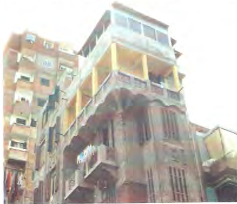
Fig.6-2, alterations and extensions to existing buildings; the quality of these extension, not only the aesthetics, but the structural as well is very much in question. A result of increasing land prices and shortage in housing supply.
