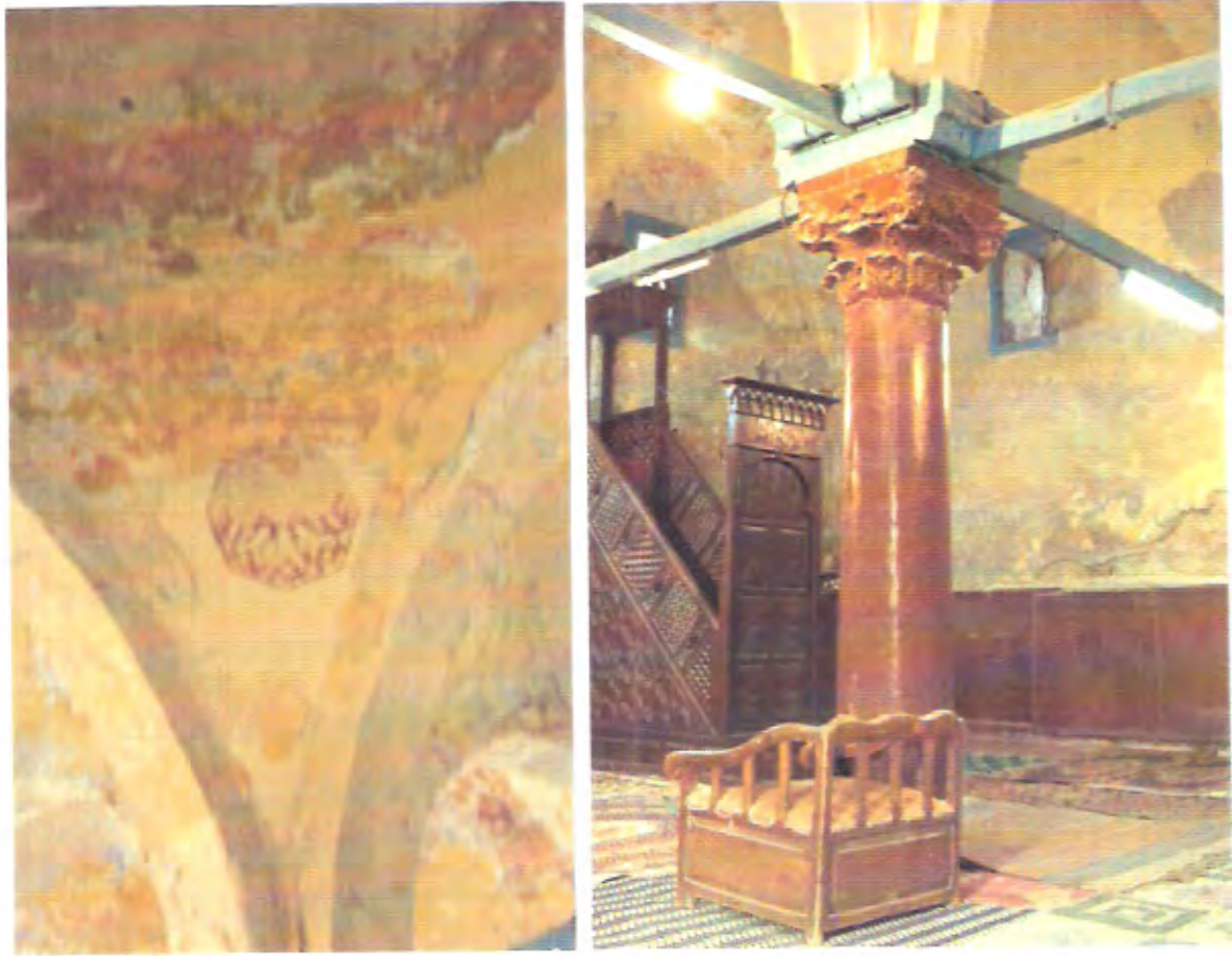
Right, the interior of the mosque, note the Minbar and the Corinthian capital; Left, the decay and deterioration of plaster and render work.
