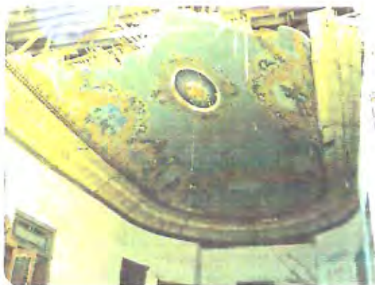
Fig.3-9, Hallabo house, Alexandria; a non listed building, which dates back to the early 19 th C. is falling down because of neglect.
