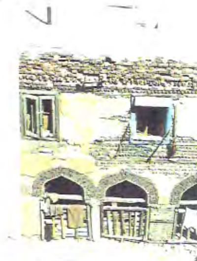
Fig.8-13, Right, inadequate rain water system causing dampness to the masonry, plaster, tiles and timber; Left, the courtyard facade; the use of brick and timber tie-beams; are in a very poor state of repair.
