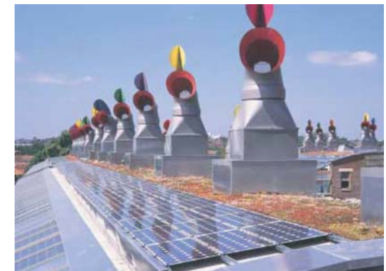
Figure 3-69: BedZED ventilation cowls, after Twinn [184]
