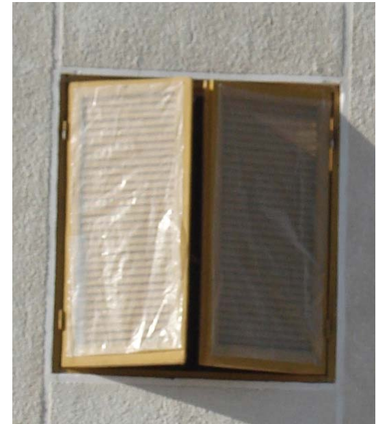
Figure 6-1: Blocking the holes of the Venetian shutters to reduce sun glare
