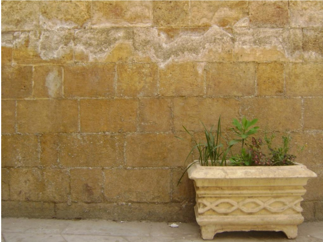
Figure 3.16 Salt layer on walls of Hassan Pasha Taher's Mosque.
