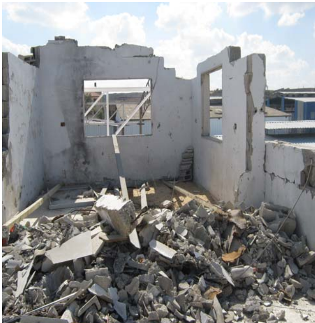
Figure 1: photo of localized failure of exterior walls, windows, roof system and columns.
