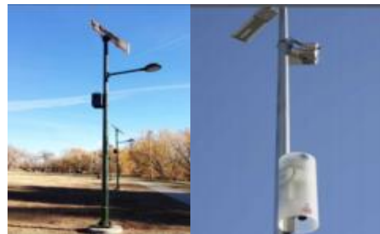
Fig. 9 - Digital additions to LED fixtures and off-grid light fixtures
