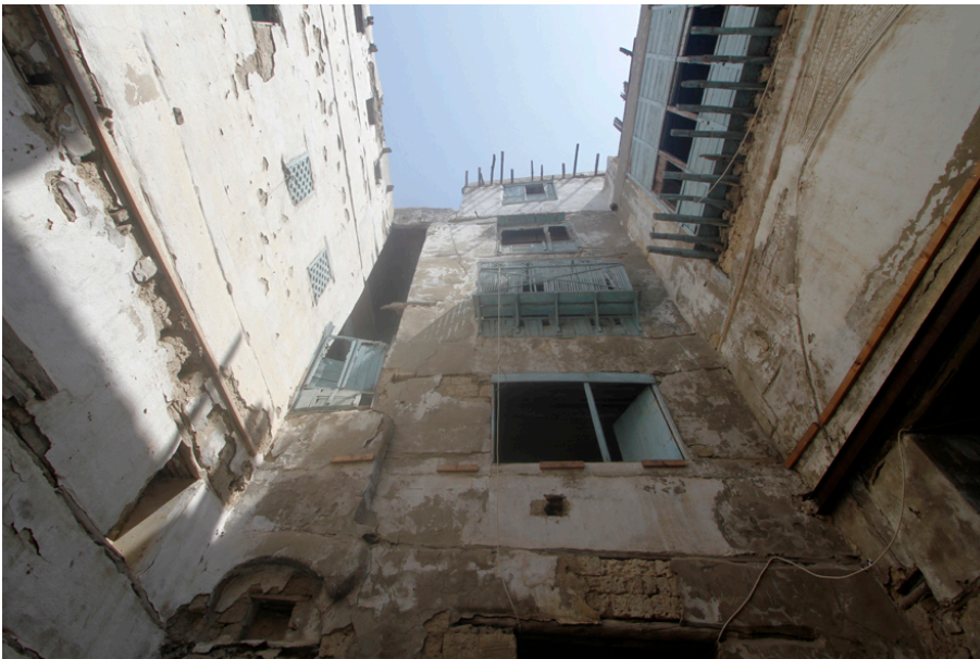
Fig. 4 Wide-angle view inside the courtyard, with the North wing to the left and the South wing with the iwan to the right, and the middle part with the wind catcher niche and roshans.
