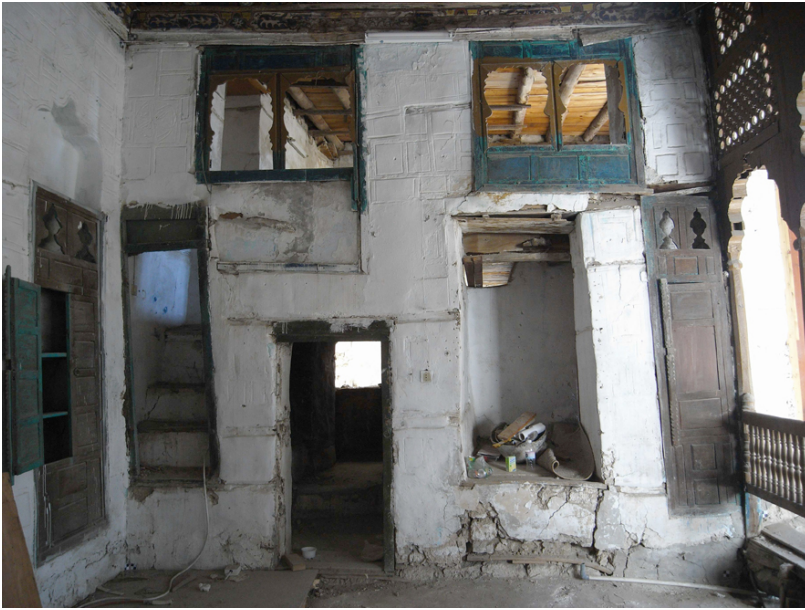
Fig. 16 South wall of room 205, the design hints to different building phases and alterations.
