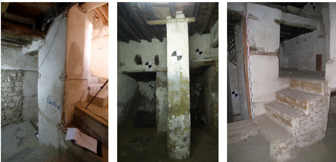
left: Fig. 8 Main staircase, between first floor landings, view of the main pillar and flights of steps. To the right (East) there was a door to the annex building.
