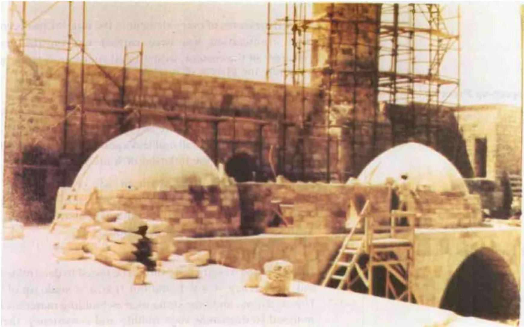
A photo showing the re-building of the southern aisle-looking over the court.
