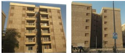
Figure (12) distortions during buildings usage - Façade's color changes
