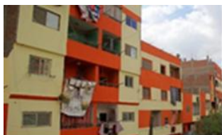
Figure (10) distortions during buildings usage - Façade's color changes
