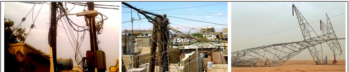
Fig(6) : Left: Deteriorated conductors and un-insulated cables in residential districts in Kerdasa and Bahteem. Right: Electrical Tower falling by storm in Alwadi-Algedid governorate, March.2014 - http://al-mashhad.com/News
