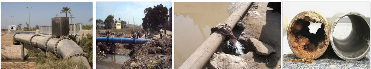
Fig(11): Pipes passing over waterways and leaking occasionally- Kafr Hakim village, Geiza.
