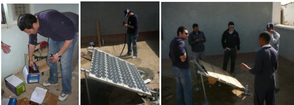
Figures 1-3: Installation of the solar system in Abu Minqar. RISE decided to recycle 30 year old panels for this project that were still working at 70 percent capacity.
