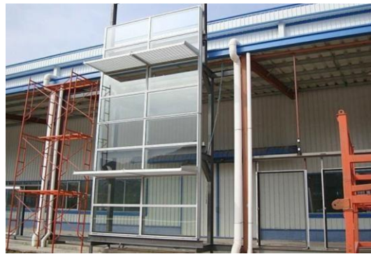
Picture (4): A unite of one floor height is ready to be fixed “Unitised Curtain Walling”.
