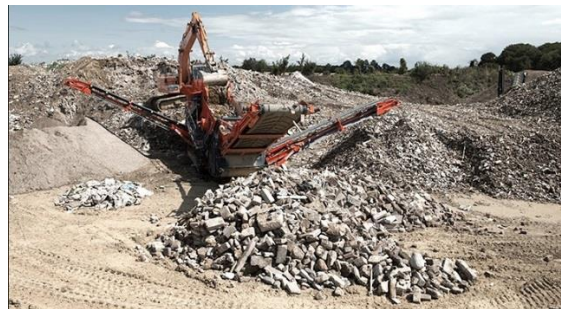
Figure 3: Equipment should have a powerful electromagnet or water flotation or an air separator system that can pull steel from concrete. [11]
